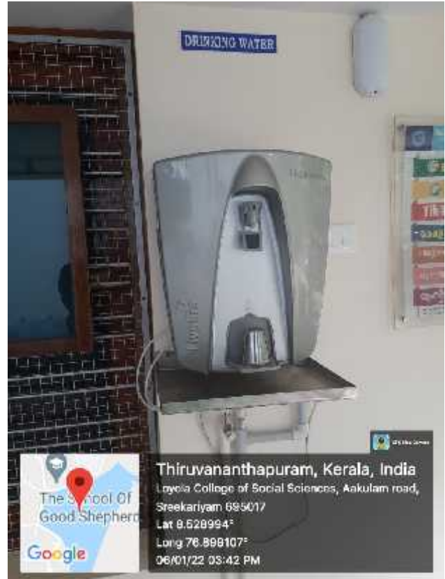
Water Purifier Installed near College Library
