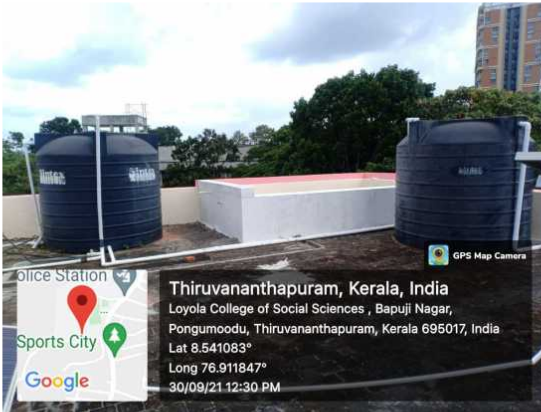
Water Tanks Installed in College Main Building
